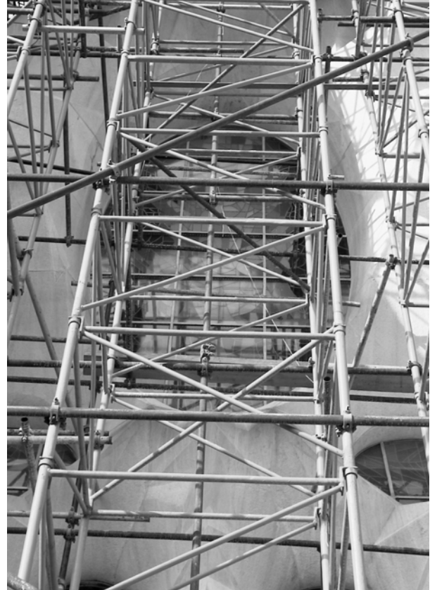
Figure 25. partially constructed window (finished and glazed at the commencement of 2001, but still site-protected and therefore not available for full-viewing at the time of publication)
