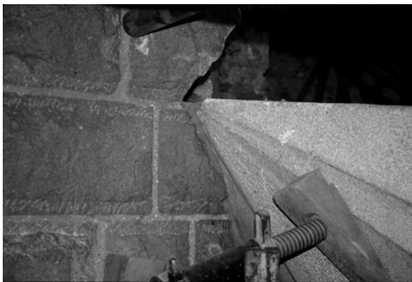
Figure 24. Close-up photograph showing of the precision given using parametric design (refer to figure 6)
